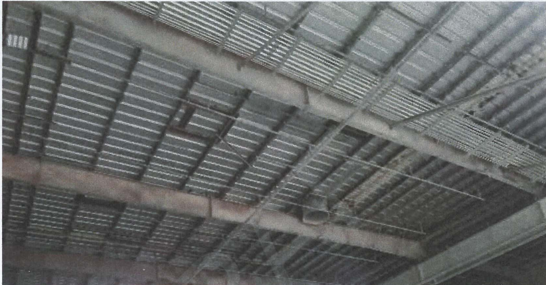
Figure 2: In the main support beams, rock pigeons can be seen roosting.
